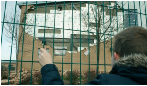
A painfully appropriate metaphor... A Scottish school, built under the PFI, in a state of collapse, April, 2016. Photographer: not known.
